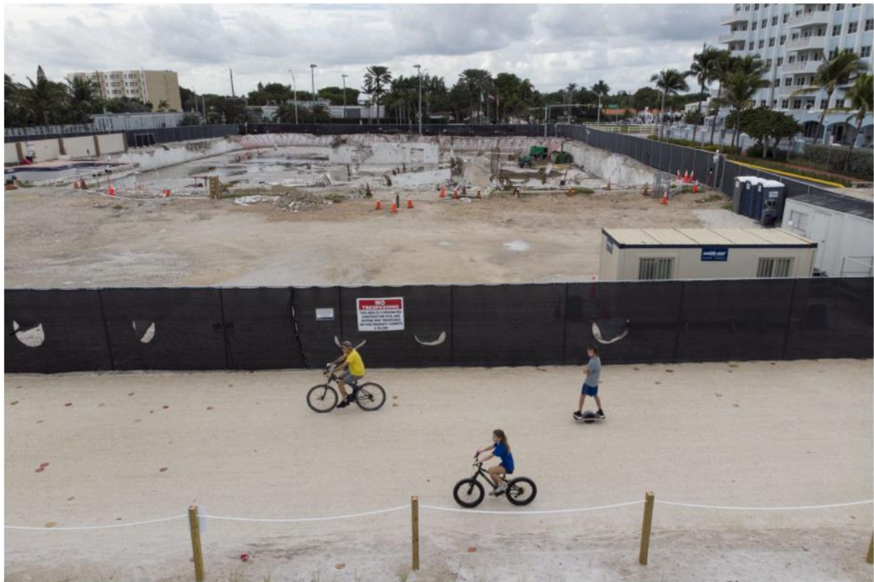
Engineers say a combination of problems likely caused the building collapse, including design flaws, poor construction and delayed maintenance.
