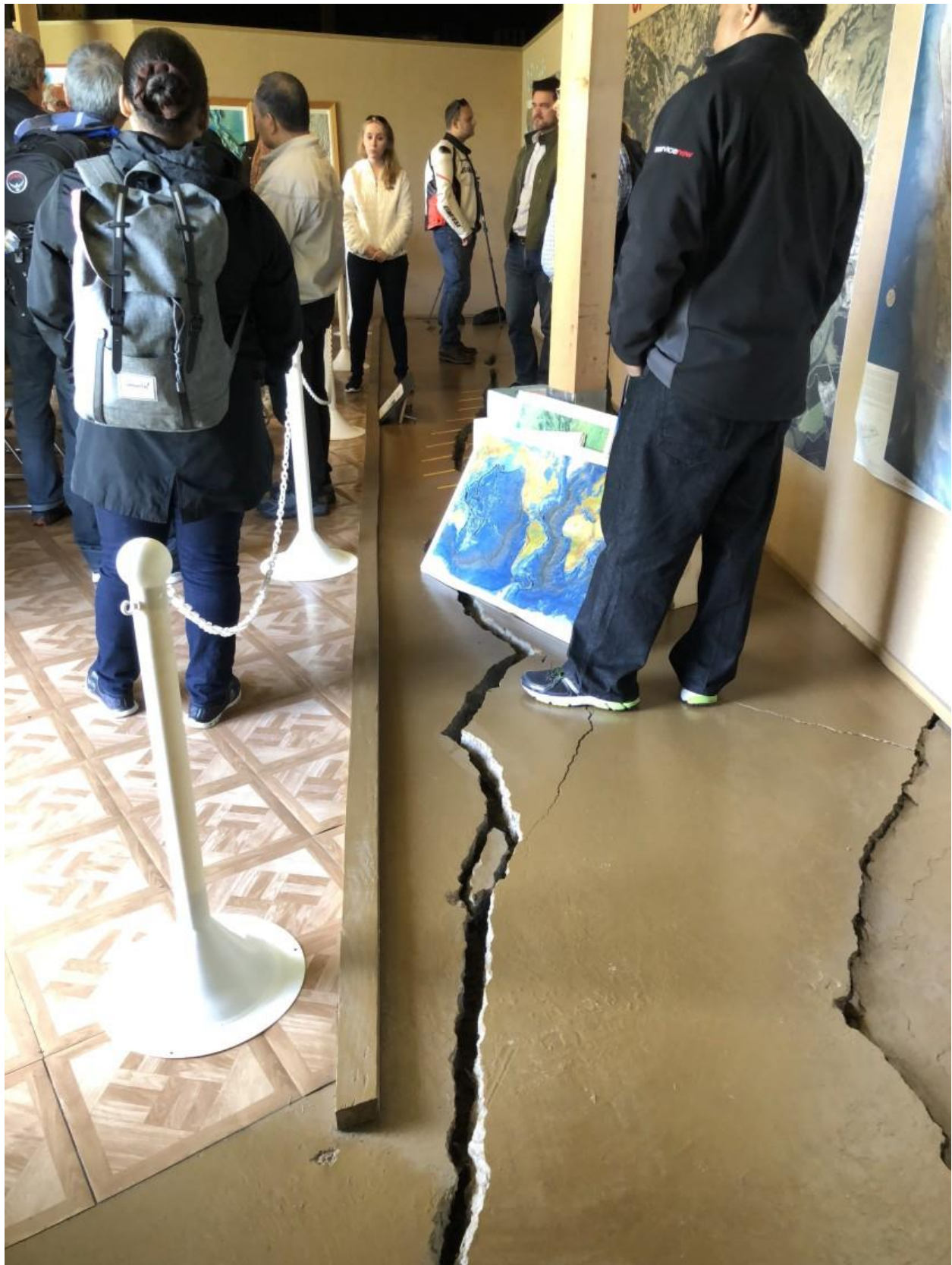
The Hayward fault is slowly tearing up the foundation of a city building in Fremont, Calif., a portion of which has been turned into an earthquake exhibit, as shown in 2018. (Rong-Gong Lin II / Los Angeles Times)
