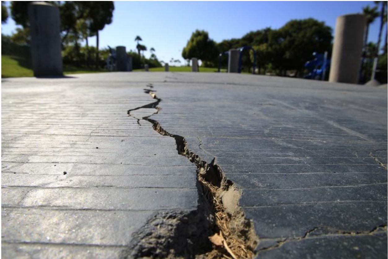
A crack splits the sidewalk at Discovery Well Park in Huntington Beach, located atop the Newport-Inglewood fault. (Allen J. Schaben / Los Angeles Times)
