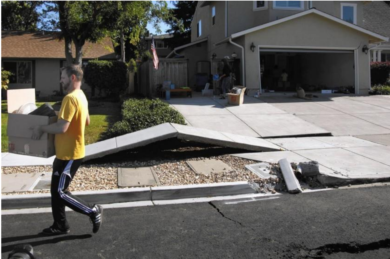
Scott Whitlock walks over a stretch of buckled sidewalk while helping his parents move out of their damaged home in 2014.. The fault line was unknown to geologists before it ruptured in Napa. (Rick Loomis / Los Angeles Times )
