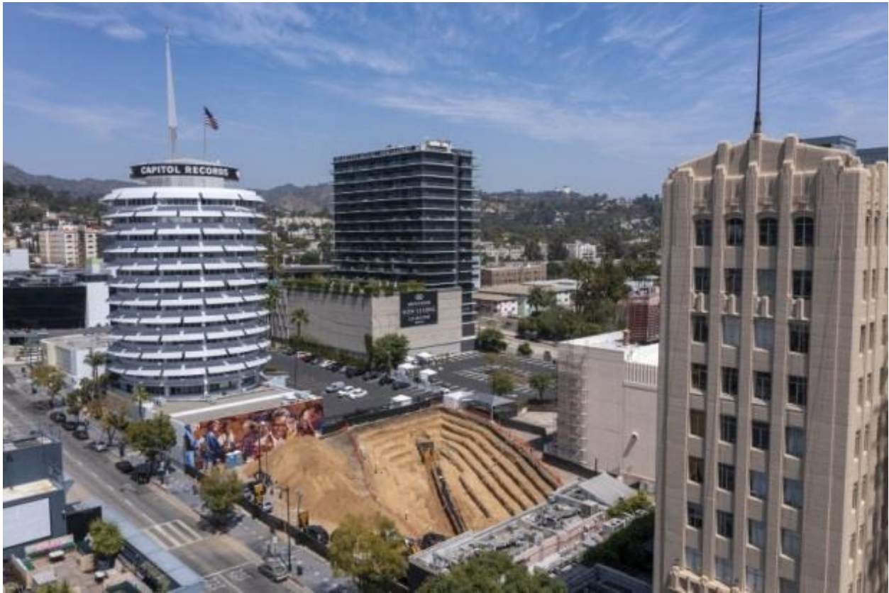
Trench at proposed Hollywood Center project. (Brian van der Brug / Los Angeles Times)
