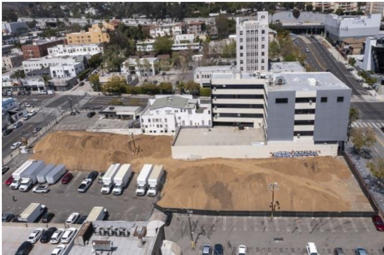
A parking lot is filled with dirt across the street from the Capitol Records building where a trench is being dug. (Brian van der Brug / Los Angeles Times)
